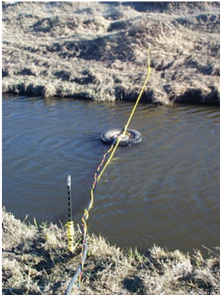
Riparian area at the time of pump installation. Photo by Dwane Morvik
